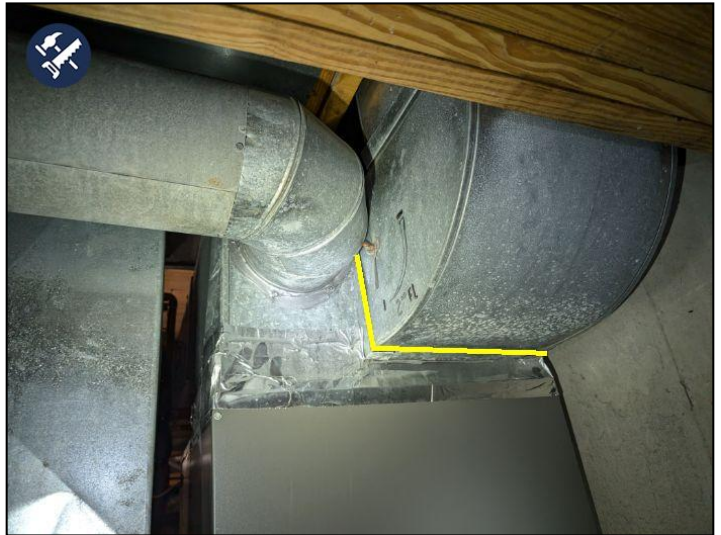
Duct tape/sealant is missing from this area. I recommend repair.
