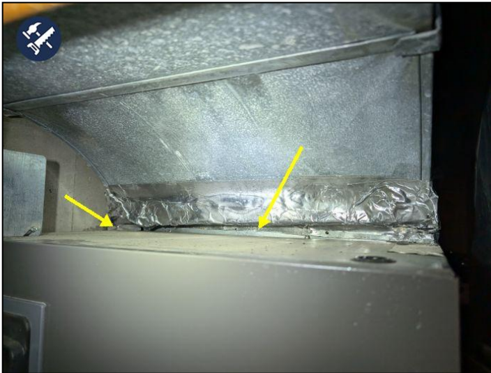
Duct tape/sealant is missing from this area. I recommend repair.
